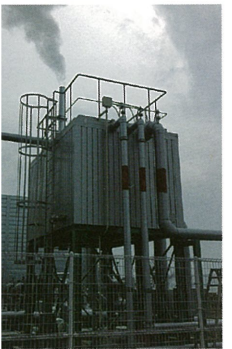
Obama Binary Power Plant
